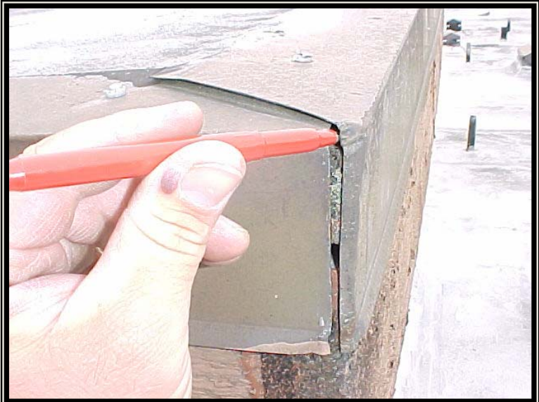
The corners in the coping on the elevator housing do not overlap, leaving an opening and potential opportunity for water intrusion.
