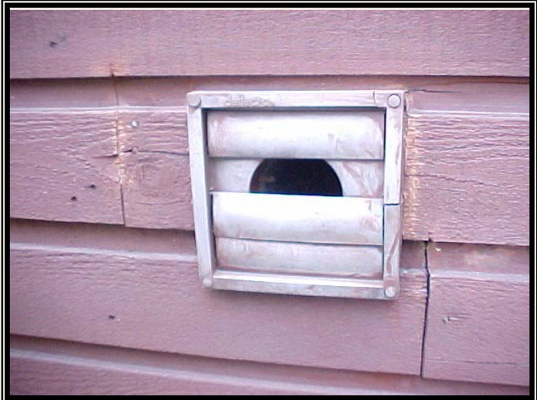
The vent ducting is detached from the vent cover. Water migrating behind the vent cover could potentially travel behind the cladding and into the interior wall cavity.
