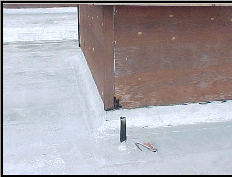
The upturned edge of the roofing membrane is exposed at this location. The building paper from the wall of the housing does not overlap the membrane and the plywood at this corner is deteriorated and decayed.
