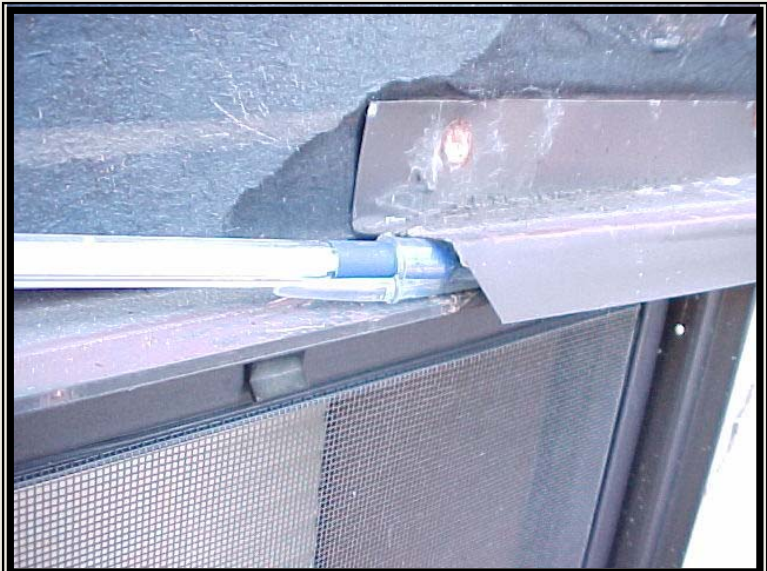
This is not a true flashing of the head of the window as the flashing does not cover the entire window head and it is not lapped shingle-fashion.
