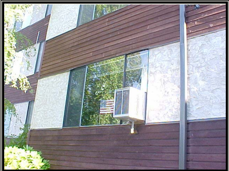
The windows in place at the Your Building Condominiums have no true expansion joint between the stucco cladding and the window frame. The perimeter is sealed however, and is observed to be in failure at every location reviewed.
