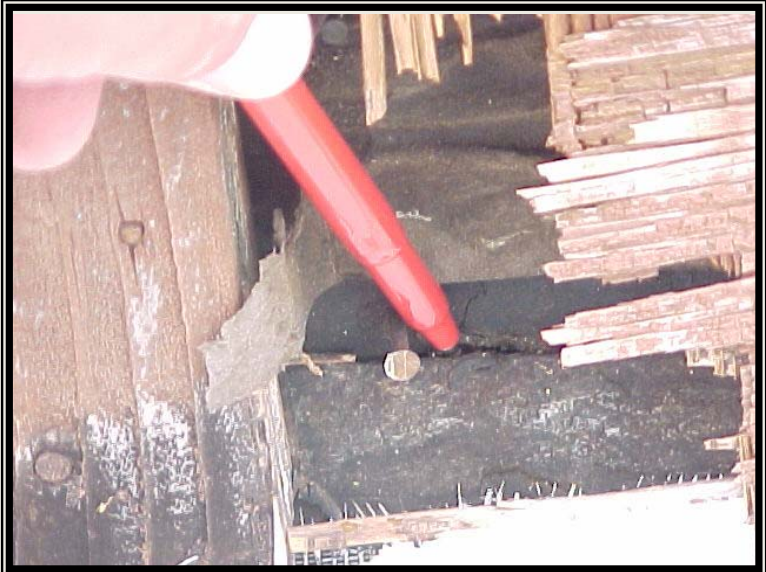
The upturned edge of the roofing membrane is exposed at this location. The building paper from the wall of the housing does not overlap the membrane and the plywood at this corner is deteriorated and decayed.
