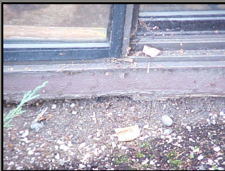
The wood trim at the sill of the window here is in contact with soil. This condition is causing the wood trim to rot/decay.
