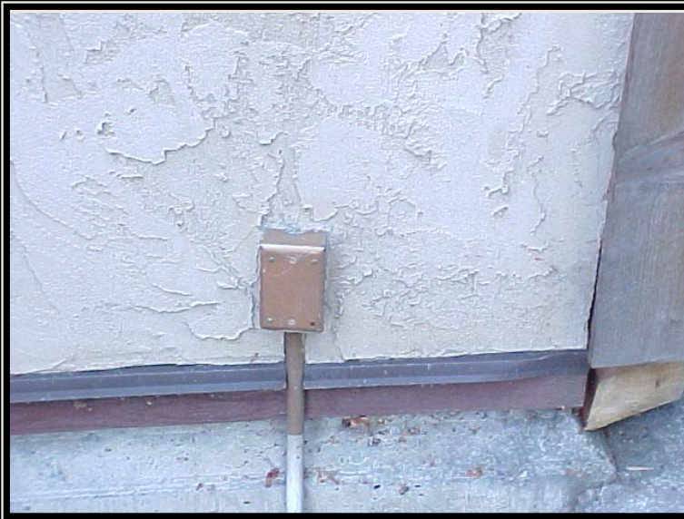
Unsealed penetrations through the cladding.
