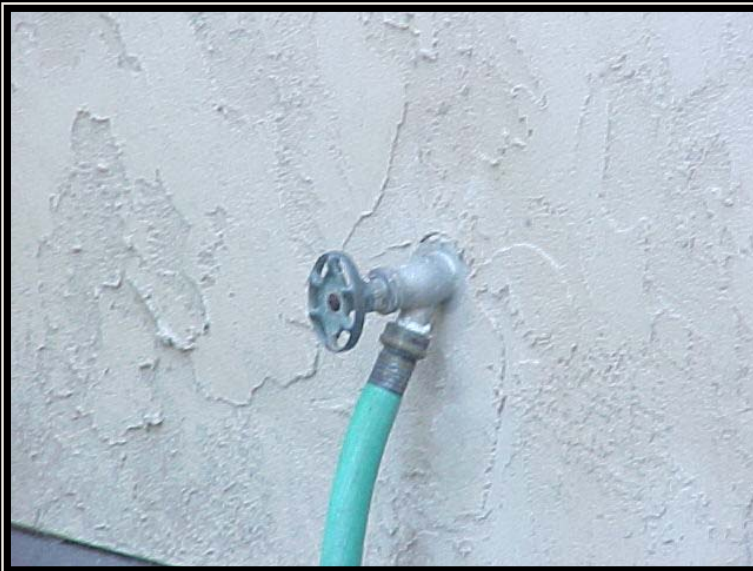
Unsealed penetrations through the cladding.
