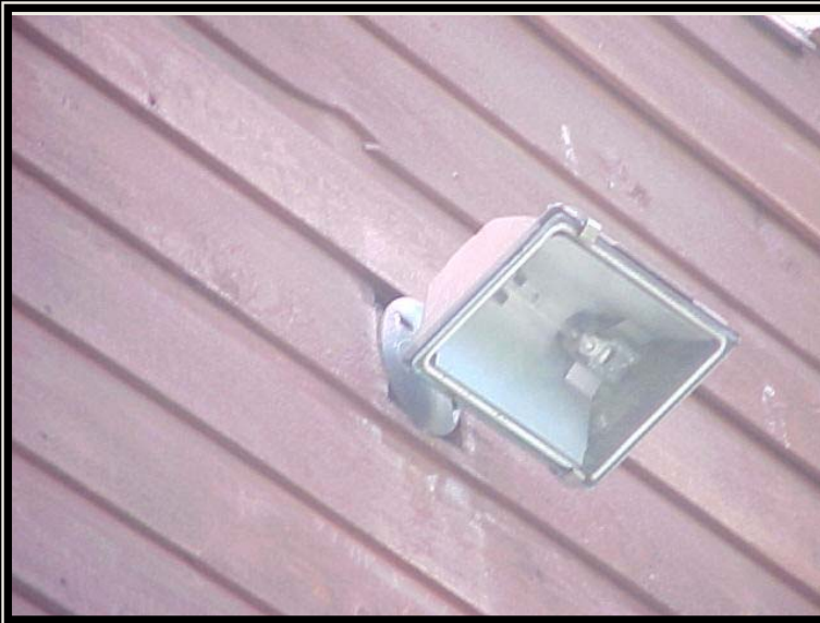
Unsealed penetrations through the cladding.
