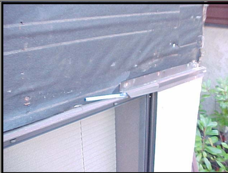
The continuance of flashing from the top of the stucco panel onto the head of the window is not imbedded in sealant at the head of the window.
